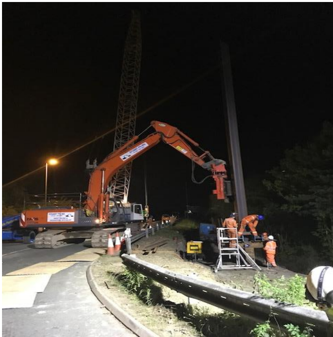
Crew on site oversee the installation of one of the sheet piles on the Over A40 Westbound
