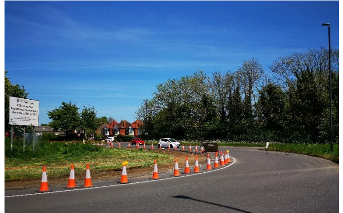
Cones will be along the white line at peak times during resurfacing
