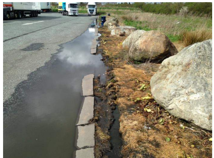
Figure 9-13 – Filter strip showing need of maintenance
