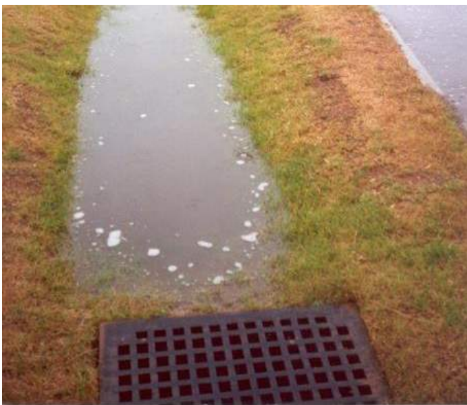
Figure 9-6 – Dry swale during rainfall showing gully outlet (SuDSnet)
