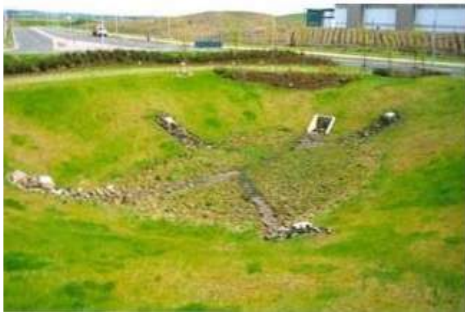
Figure 10-1 – SuDS pond with inlets and outlet
